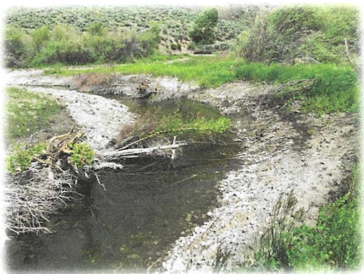
New River Channel on the Lemhi River showing wood placement and wood fish habitat.
