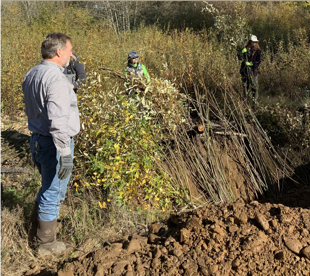
Volunteers lay in willow cuttings prior to be anchored into the streambank with heavy equipment. SWC Engineer Bill Lillibridge supervises. (courtesy KSSWCD)
