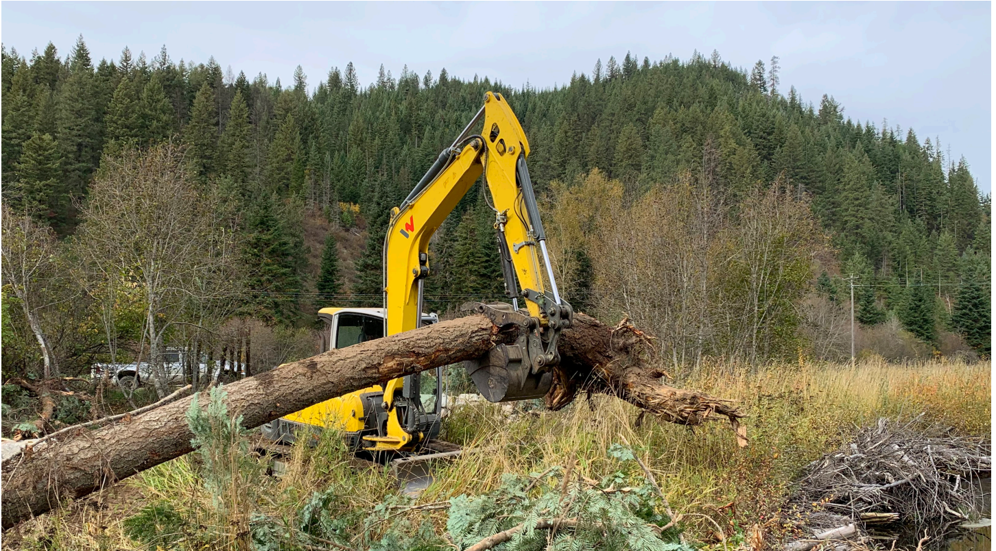
Contractors place a root wad on Wolf Lodge Creek to anchor the streambank on Steve and Janet Funk's Edgecreek Tree Farm near Lake Coeur d'Alene (photo courtesy Kootenai-Shoshone SWCD).
