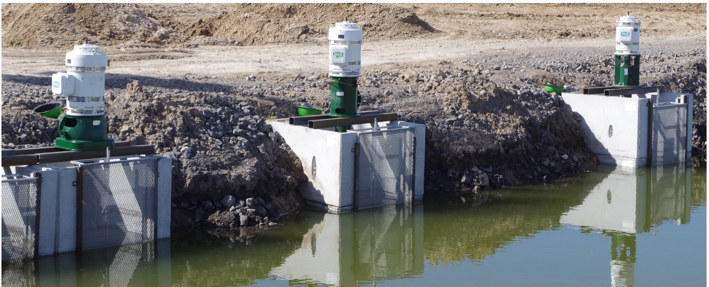
New water pumping stations fitted with Variable Frequency Drives will run more efficiently than North Side Pumping’s old system, saving water and energy. Each pump serves a total of 30 producers in the project area. (photo by Steve S.)
