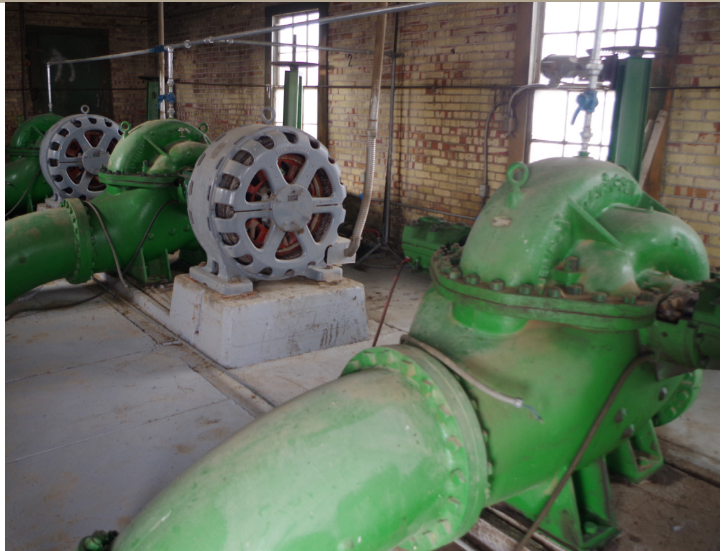
North Side Pumping will retire these old pumps that date back to 1929. (photo by SS)
