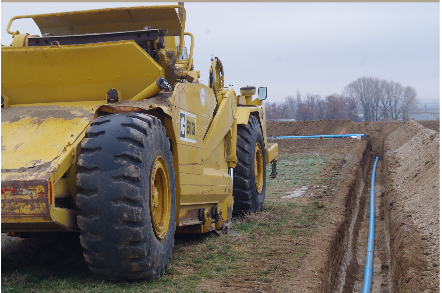
Butte Irrigation dug deep trenches for the pipeline installation in an area that locals say has fewer rocks under the ground than many areas in the valley, making it easier-going for the contractor. (Photo by Steve Stuebner)
