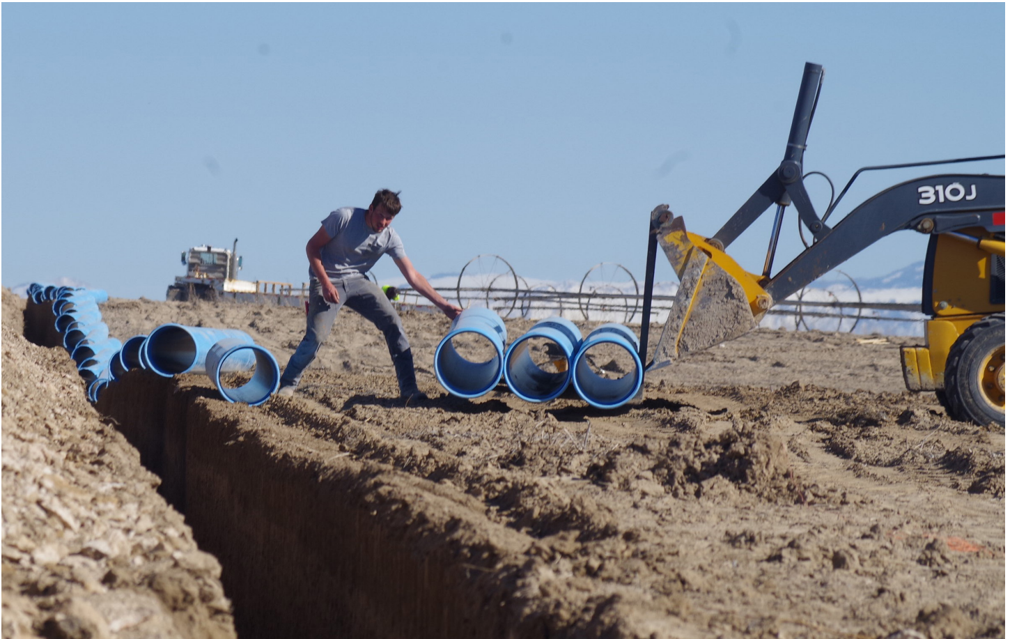
Butte Irrigation employees install PVC irrigation pipe on a farm served by North Side Pumping Co. in Hazelton. The contractor installed 88,000 linear feet of buried pipeline for the irrigation efficiency project. (photo by Steve Stuebner)
