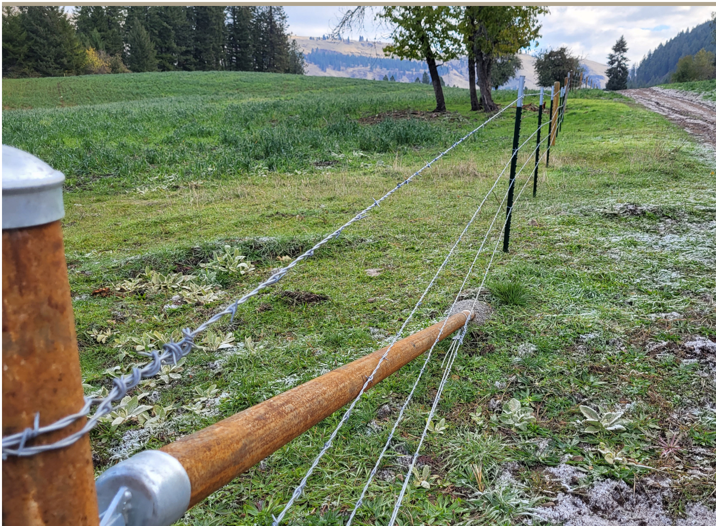
New 4-strand barbed-wire fencing on Neil Uptmor's farm and ranch. (photo by Eileen Rowan/SWC)
