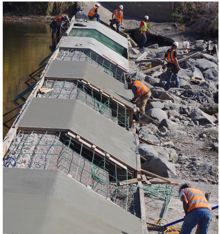
Braun-Jensen crew smooths out concrete on a warm October afternoon, perfect conditions for the concrete pour. (photo by Steve Stuebner).
