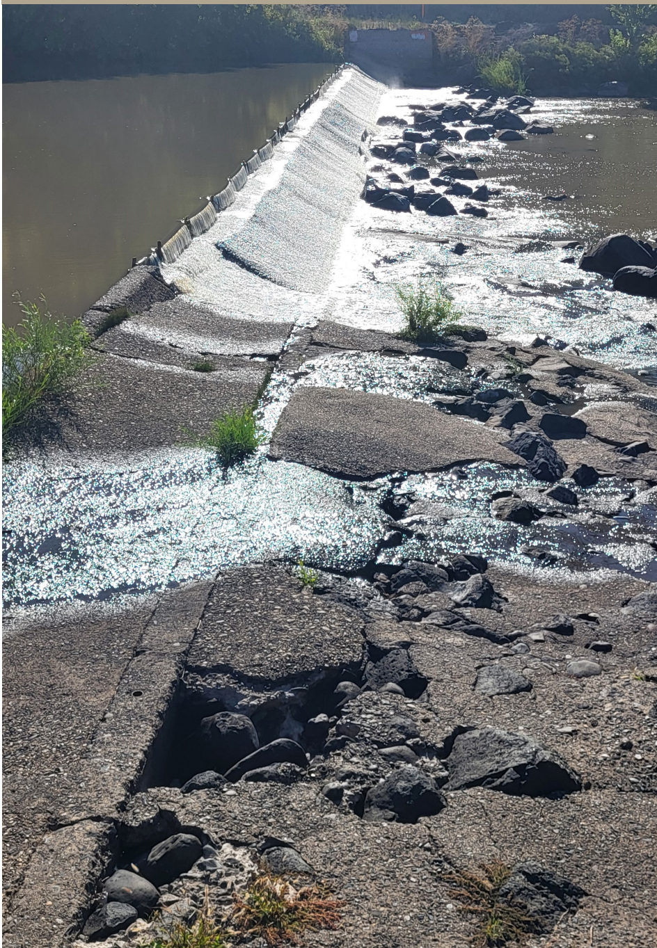
Pre-construction, cracks and deterioration can be seen in the diversion dam structure. (photo by Meghan Brooksher/SWC)
