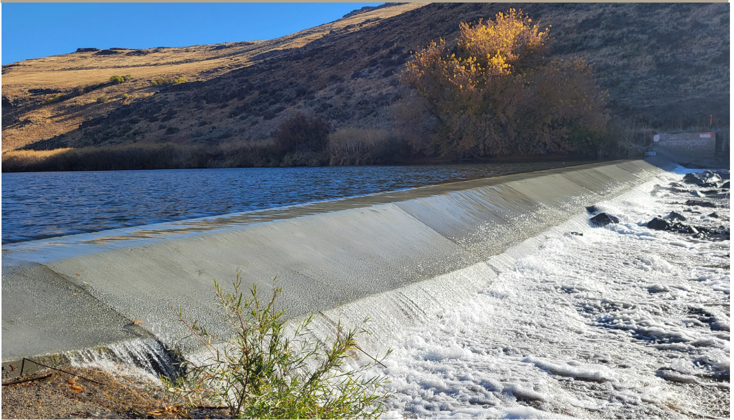
The finished product: Galloway Diversion Dam, with its new concrete finish gleaming in the early-morning sunlight. (photo by Meghan Brooksher/SWC)
