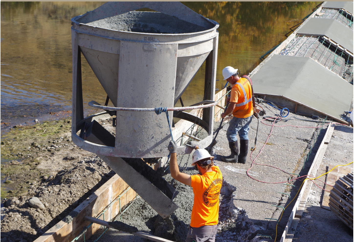
Braun-Jensen crew pours concrete into forms on the front face of the Galloway Diversion Dam on the Weiser River. The rehabilitation work will ensure that Galloway can serve local farmers for many years to come. (photo by Steve Stuebner)
