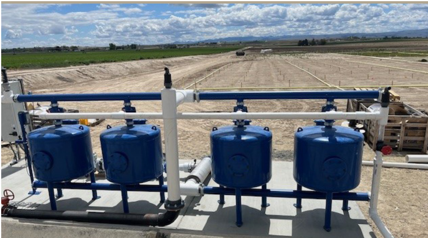
Drip irrigation system being installed on a mint field at the Chris Gross farm in Canyon County. (photo by Stan Hays)
