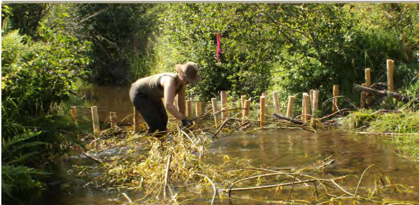
A volunteer weaves willows through a series of posts to build a BDA on the East Fork of the Potlatch River. Using local woody materials saves time and money when building BDAs and PALS. (photo by PCEI volunteers)
