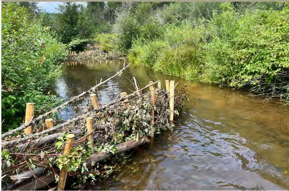
PALS structure installed on the East Fork of the Potlatch River will slow down the current and deflect flow away from the streambank, while providing hiding and rearing habitat for fish. (photo by Annie Connor, Clearwater SWCD)
