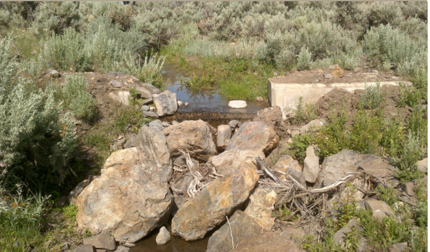
New check dam installed by the Butte SWCD as part of a Sage Grouse Action Team grant. (photo by Butte SWCD)
