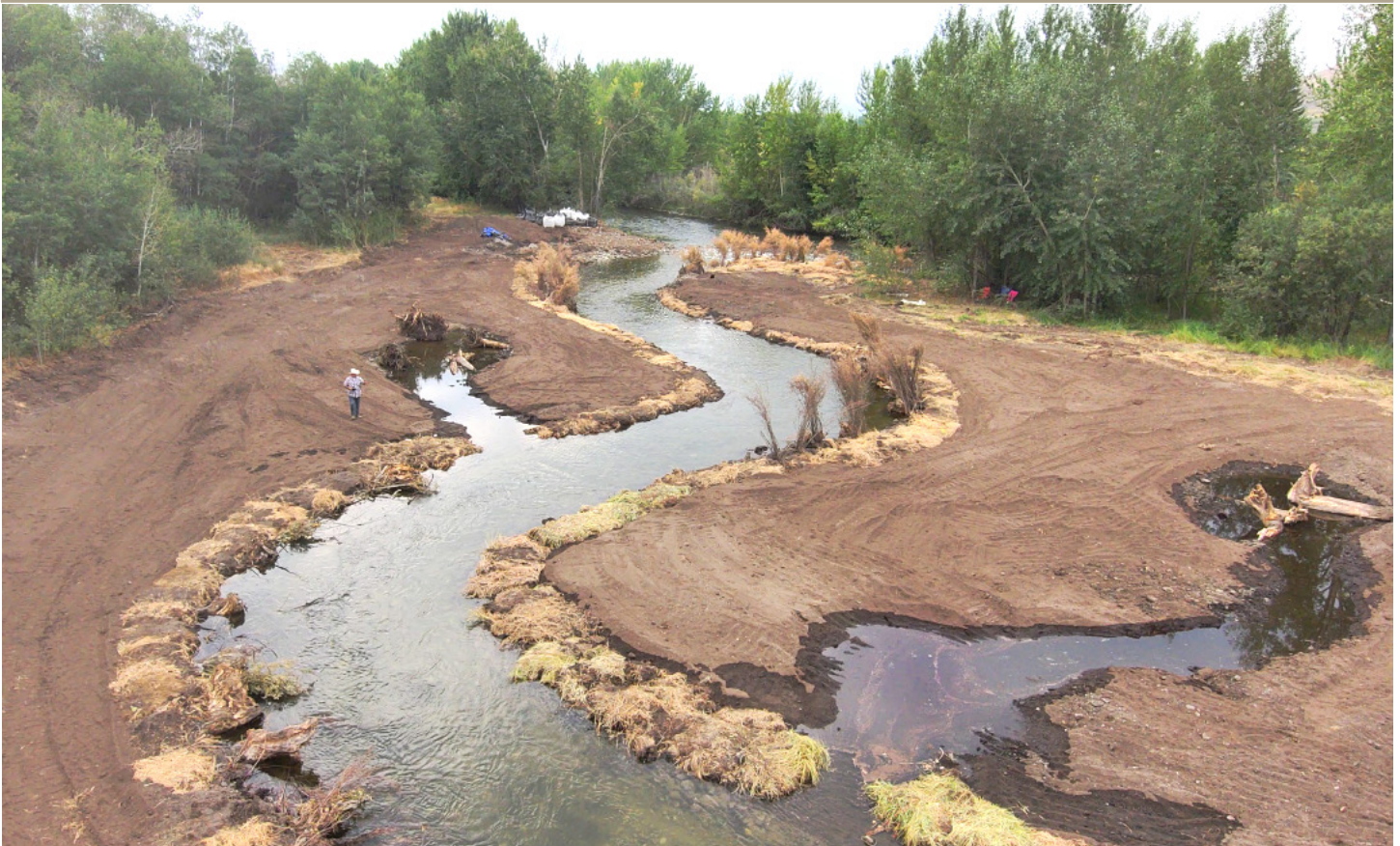
New side-channel under construction near Tendoy, Idaho, on the Lemhi River. (Courtesy Lemhi SWCD)
