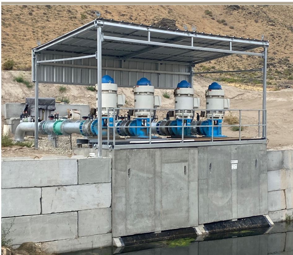
New pump station on the Snake River for West Indian Cove Water Co. was funded by NRCS, an Aging Infrastructure Grant from the IWRB, and a WQPA grant. Total project cost was $1.6 million. (Photo courtesy Dale Hooley)
