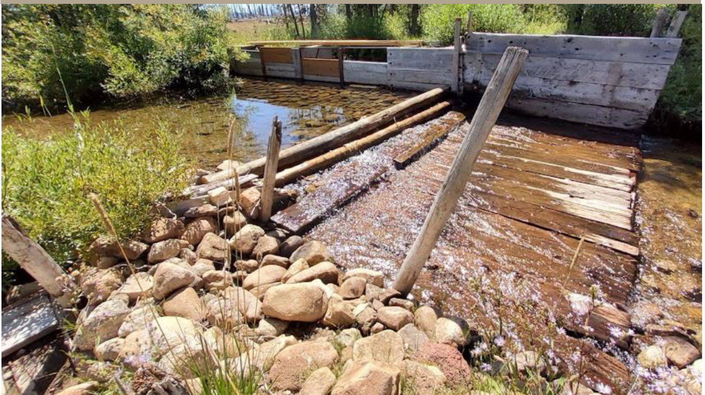
The previous irrigation diversion on the Cape Horn Ranch was difficult for native fish to navigate, especially at low flow. (Courtesy Custer SWCD)
